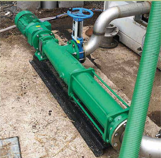
BIOMASS TRANSFER PUMP Flow – 40 m³/hr, Pressure – 3 bar
