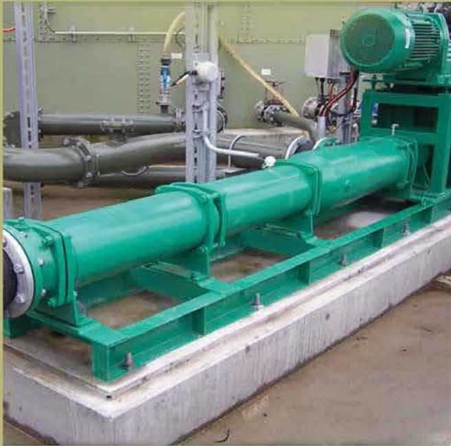
DIGESTATE TRANSFER PUMP Flow – 75 m³/hr, Pressure – 10 bar
